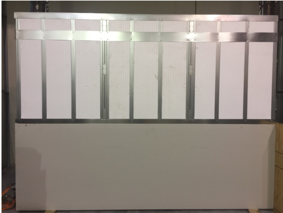
Figure 5: The exposed face prior to the first layer of gypsum being completed.
